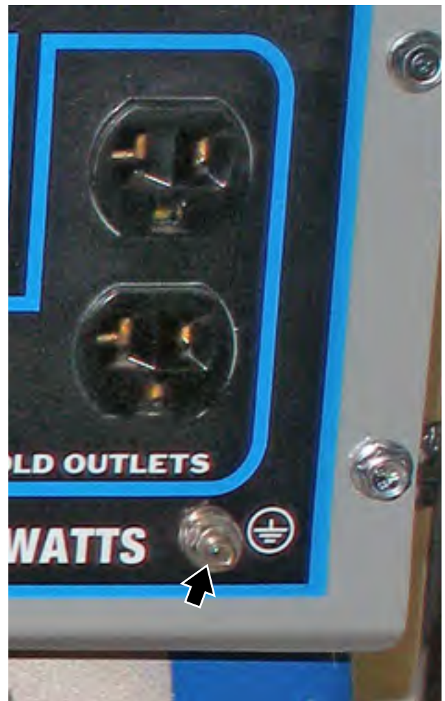
Figure 12 – Ground Terminal on the Control Panel
